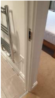
Captured (certified by inspector): 01/04/19 Added: 04/04/19
