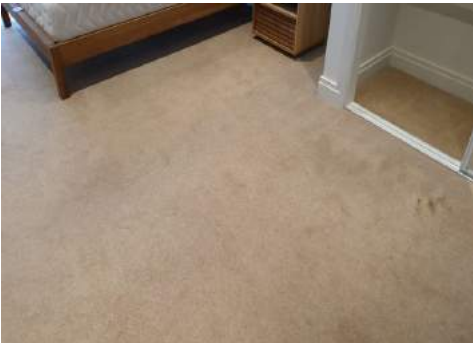
Captured (certified by inspector): 01/04/19 Added: 04/04/19
