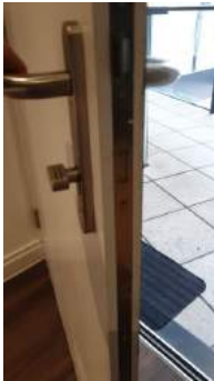
Captured (certified by inspector): 01/04/19 Added: 04/04/19
